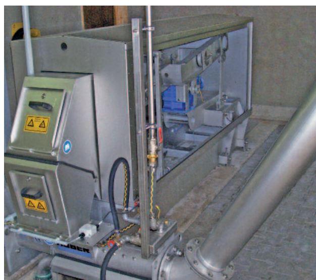
Channel installation of a HUBER Curved Bar Screen CurveMax® with downstream wash press
