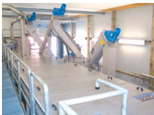
Odour-encased screenings discharge from the HUBER Complete Plant ROTAMAT® Ro5
