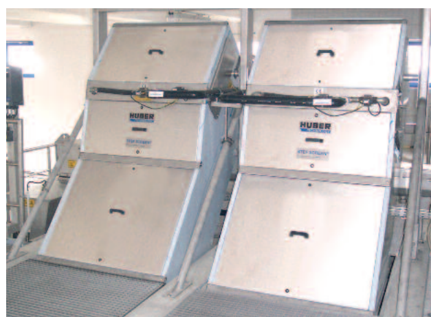
Two HUBER Fine Screen STEP SCREEN® SSF units installed in parallel channels
