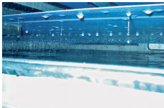
View into the filtrate chamber
