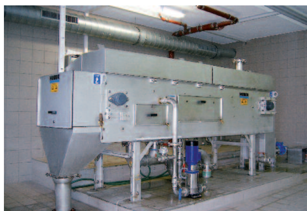
Belt washing with filtrate water as spray water
