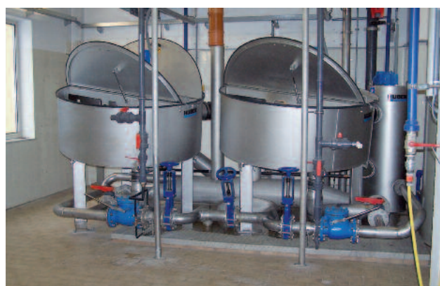
Zwilling-Installation in engem Raum
