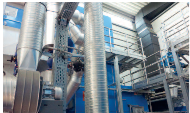
Innovative concept of decentralised sludge utilisation by generation and use of thermal and electrical energy
