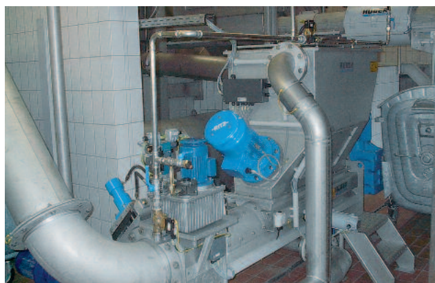
Maximum washing and dewatering results
